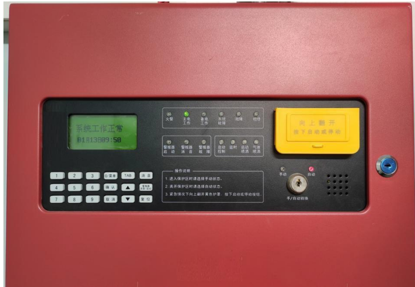
Rated service condition of the fire alarm controller
